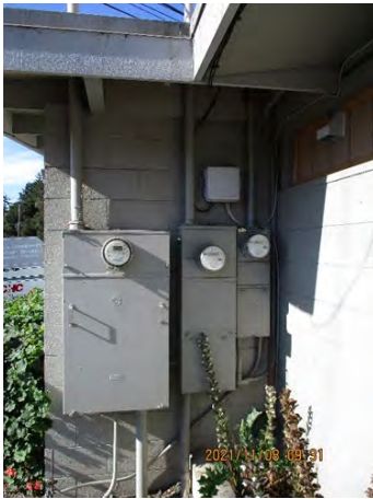
PG&E service nos. 1, 2, and 3
