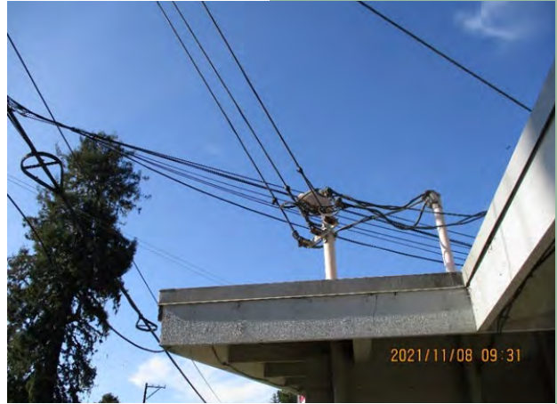
Electric service hodge-podge of wiring
