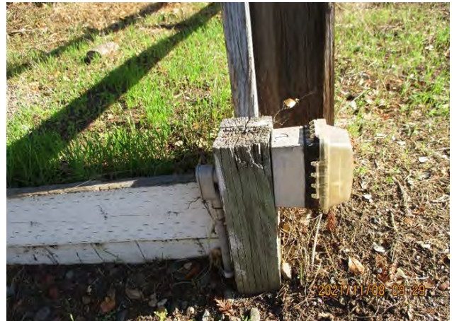
Non-compliant exterior outlet
