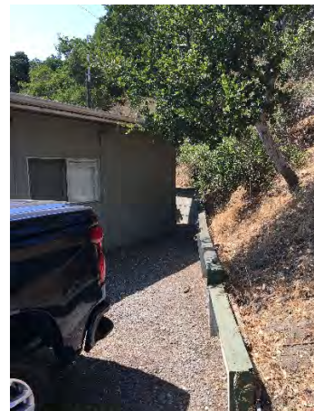
Debris wall behind facilities
