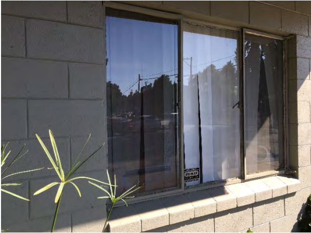
Window doesn't close properly
