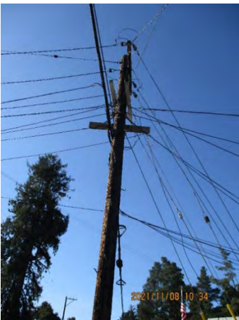
PG&E service pole
