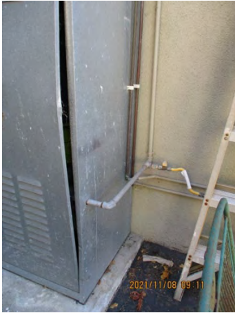
Non-compliant gas connection
