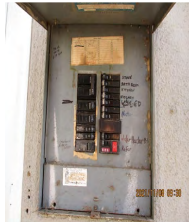
Electrical distribution panel
