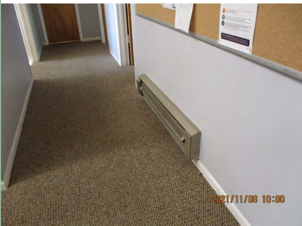
Non-working wall heater
