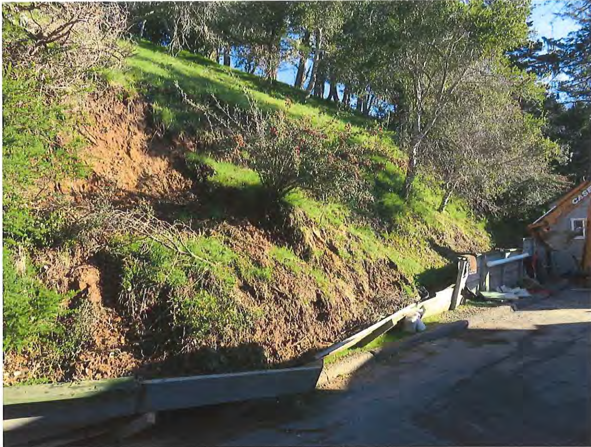
Figure 4: View northeast of failure of cut slope. Note proximity of building in back to cut slope and failure of wood wall. Trench T-1 was excavated near the building, Trench T-2 was excavated in the slide, and Trench T-3 was excavated just left of the sight of the picture.
