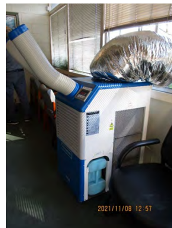
Evaporative cooler at CHC
