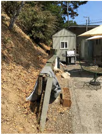
Failing debris wall
