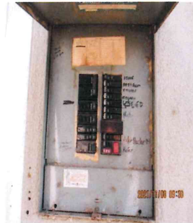
Electrical distribution panel
