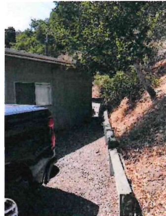
Debris wall behind facilities
