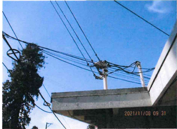
Electric service hodge-podge of wiring
