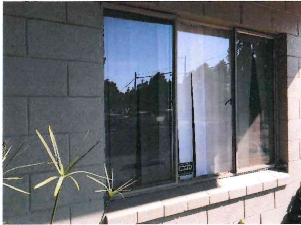
Window doesn't close properly
