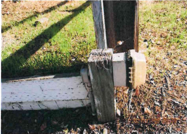
Non-compliant exterior outlet
