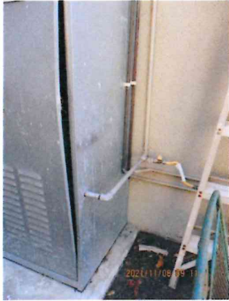
Non-compliant gas connection
