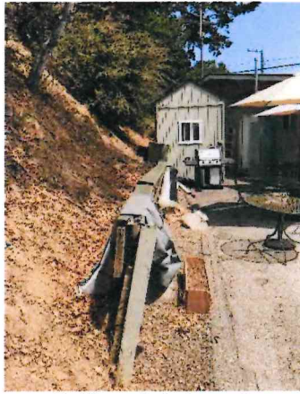
Failing debris wall
