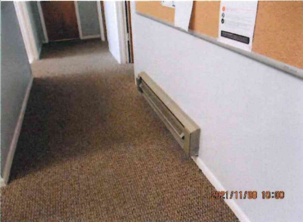
Non-working wall heater
