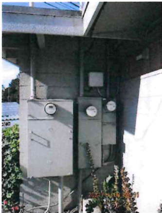
PG&E service nos. 1, 2, and 3
