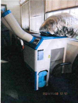
Evaporative cooler at CHC
